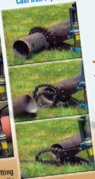
Cast Iron Pipe
