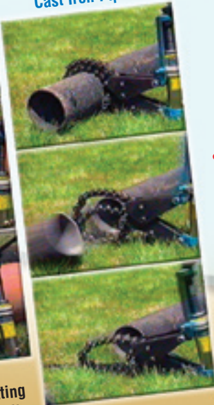
Cast Iron Pipe
